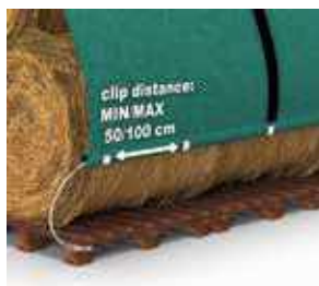
A. Secure the fabric to a metal pipe with steel clips at a distance of min 50 and max 100 cm, depending on the wind speed.
